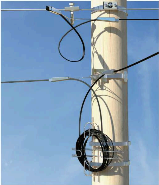
FIBER OPTIC CABLE
