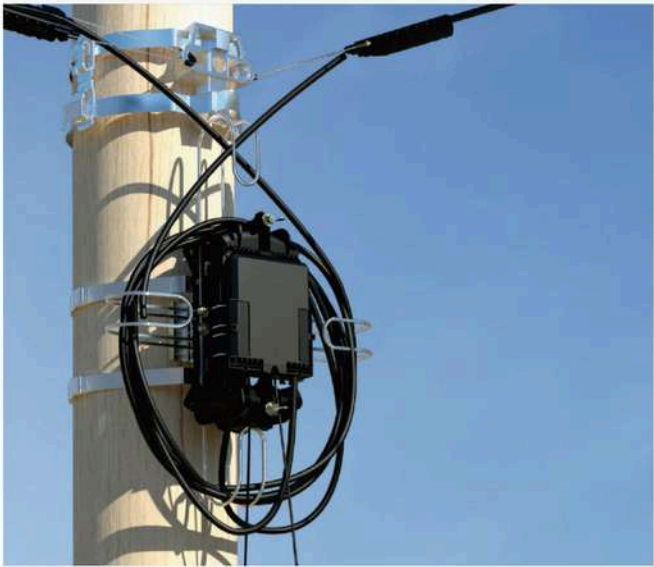
FIBER OPTIC SPLICING & TERMINATION SYSTEM
